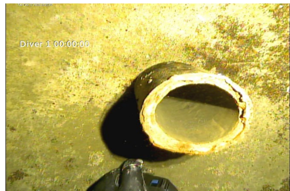
(#23) Drain with Rust Nodules
