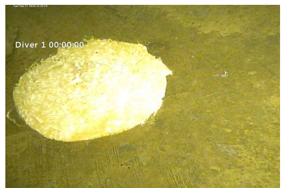
(#24) Previous Epoxy Floor Repair
