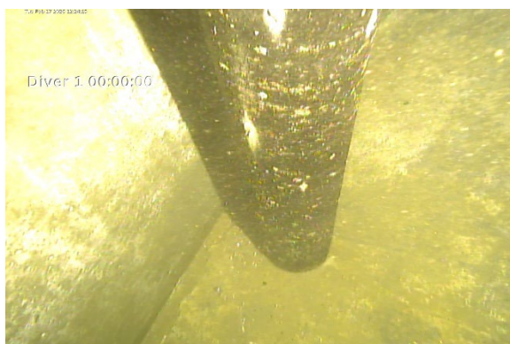
(#21) Inlet Pipe with Rust Nodules
